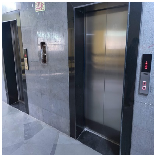
Lift Facilities at Hostel
